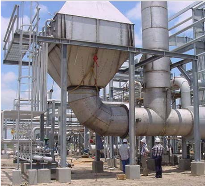
Flue Gas Heat Exchanger (EX101)
